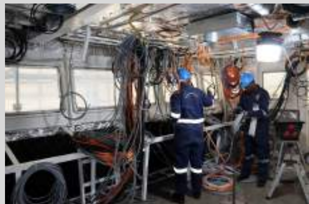
© KSL- Cable dressing in the Bridge for KNS Shupavu of the @KSL- kdfinfo at Mombasa Shipyard. KSL is committed to delivering the vessel within a short time and using minimal resources which will, in the end, go a long way in enhancing safety and security of Kenyans
